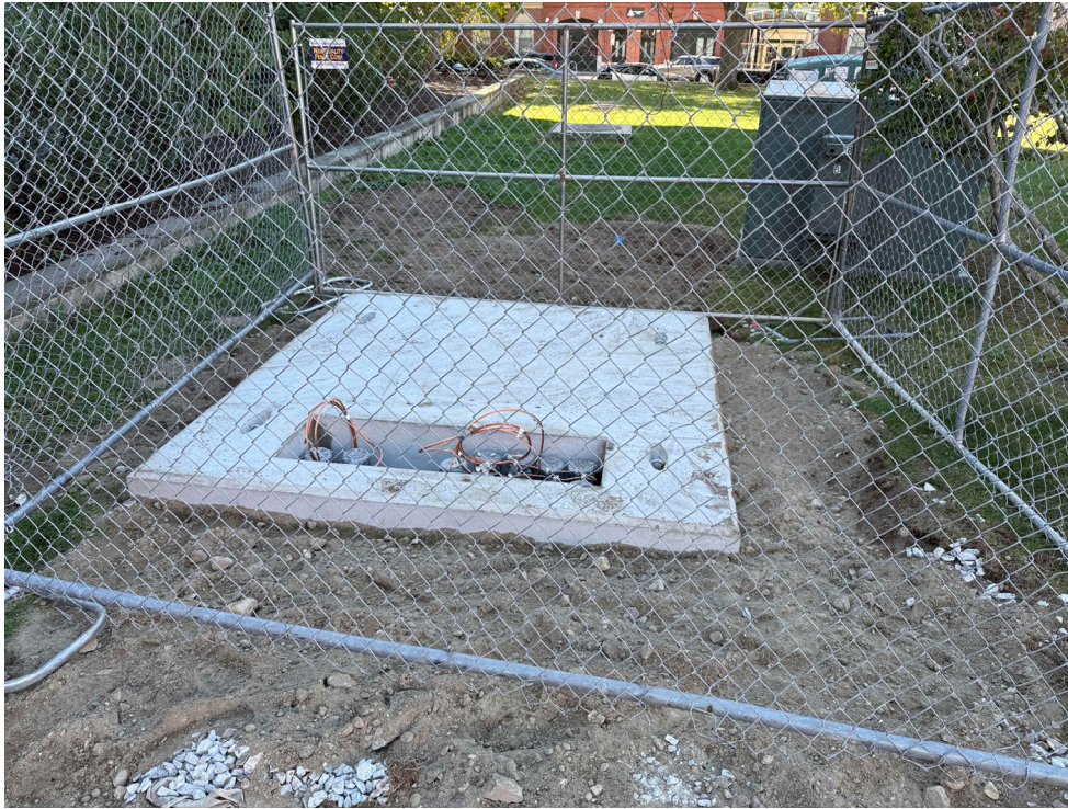
Electric transformer pad, 10/06
